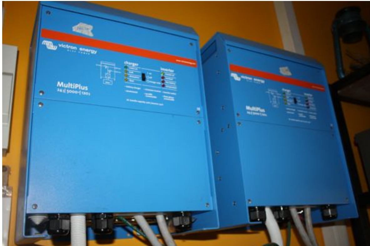
Fig 3. 2 x inverter chargers
